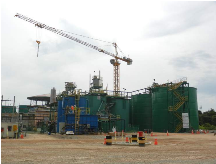
Figure 17.1.3 CIL and leach tanks (June, 2012).
