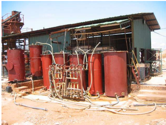
Figure 5.3 Heap leach tanks
