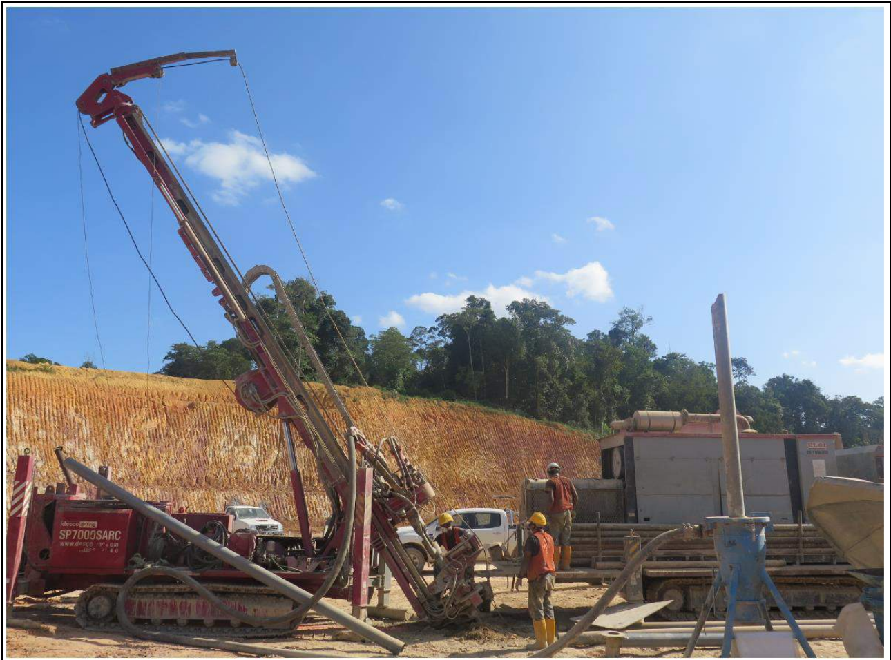
Figure 10.3 RC drilling by contractor at Buffalo Reef (photo taken during 2016 Snowden site visit)
