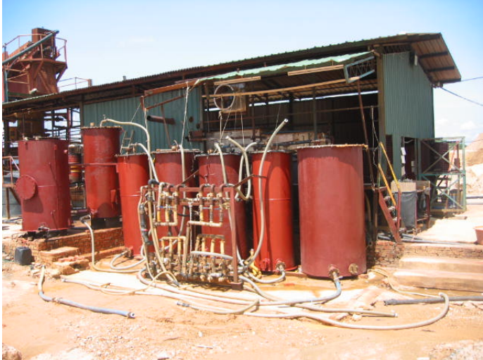
Figure 5.3 Heap leach tanks
